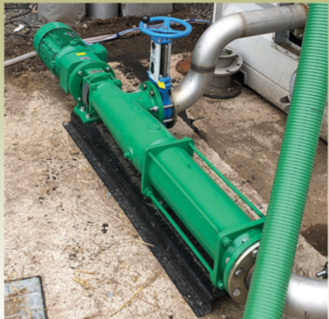
BIOMASS TRANSFER PUMP Flow – 40 m 3 /hr, Pressure – 3 bar
